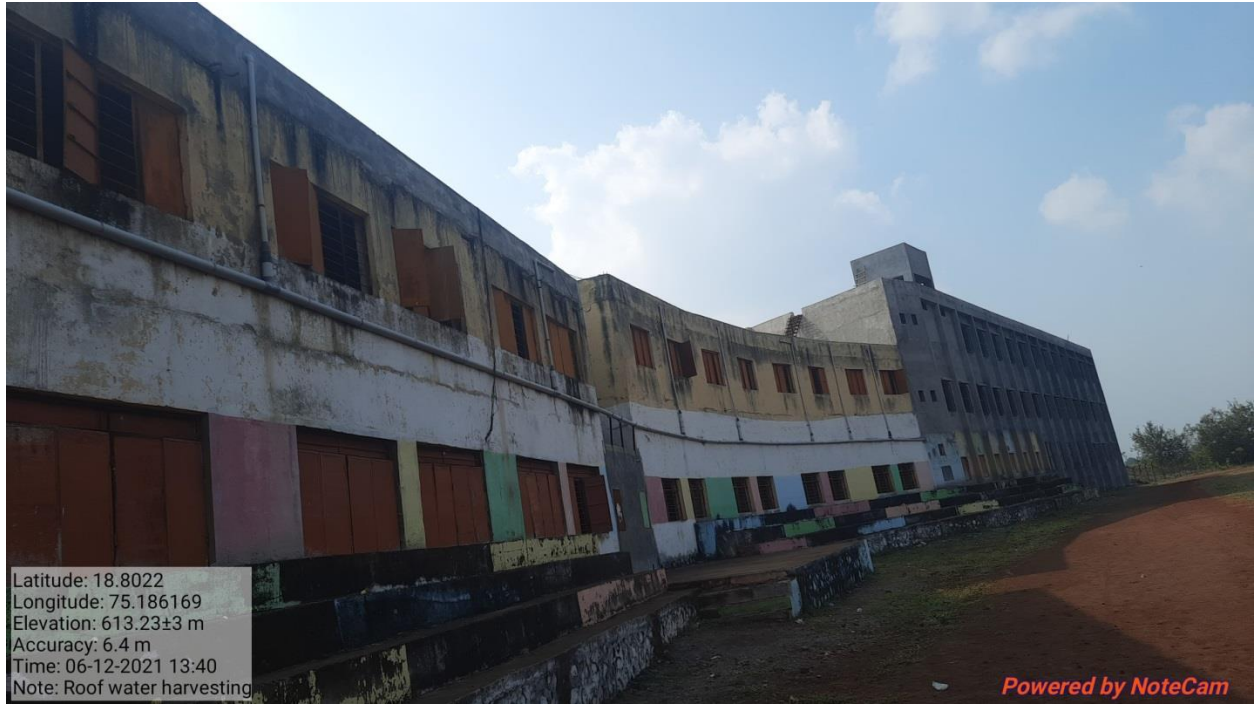
Roof Water Harvesting
