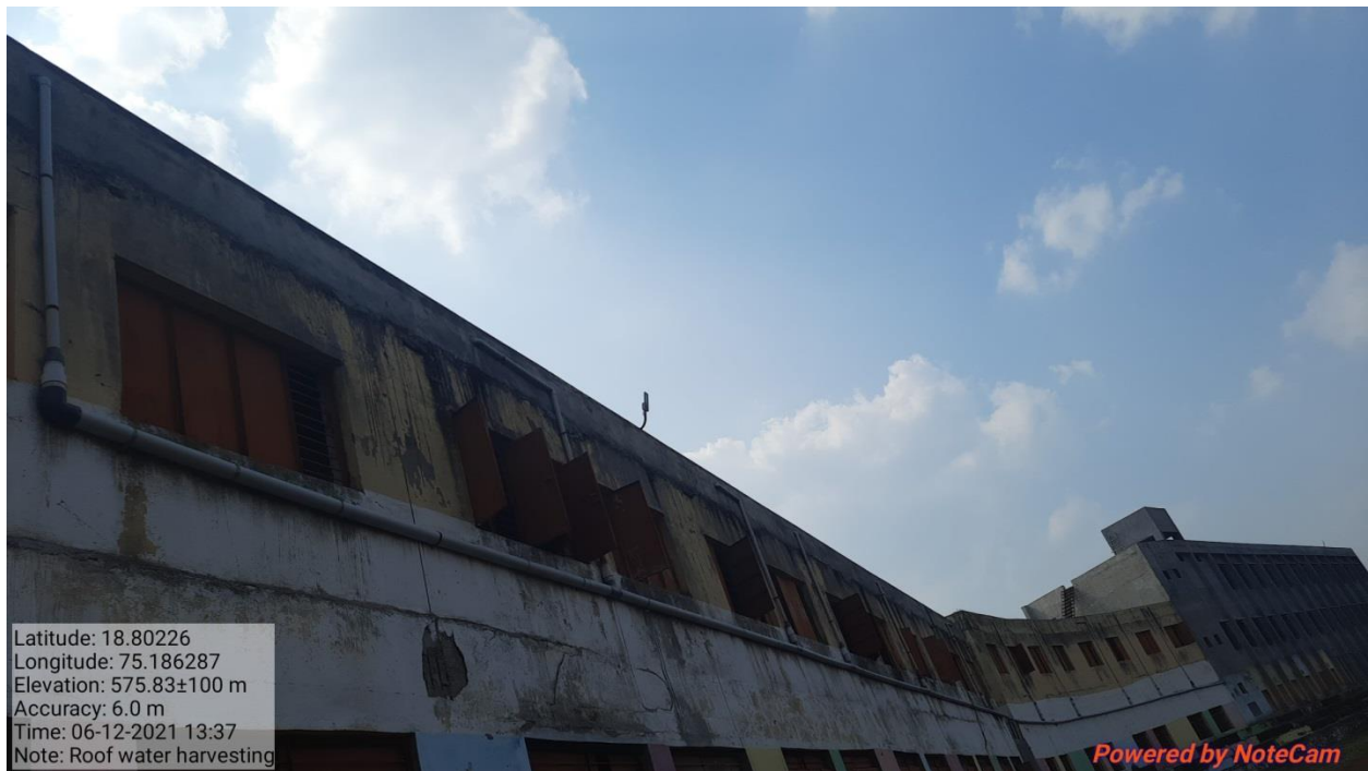
Roof Water Harvesting
